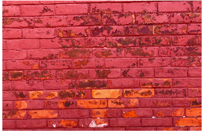
▲ Peeling paint on brick
