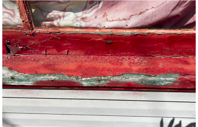
▲ Peeling paint on wood
