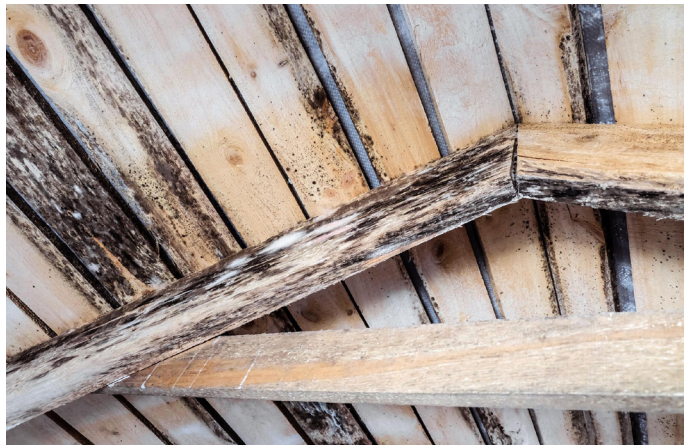
^ Wood rotting due to humidity and growth of molds
