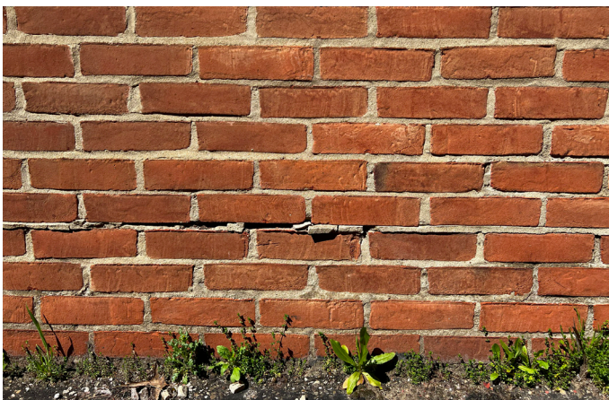
^ Mortar joints starting to deteriorate
